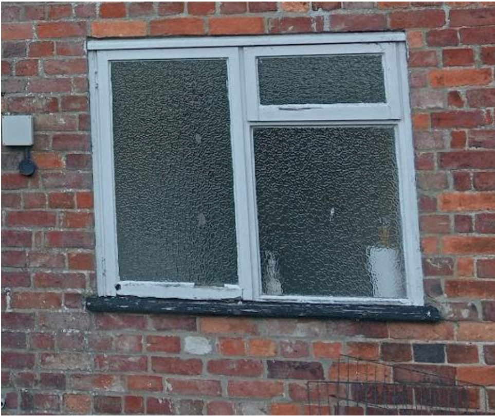
Deteriorating timber windows to rear
