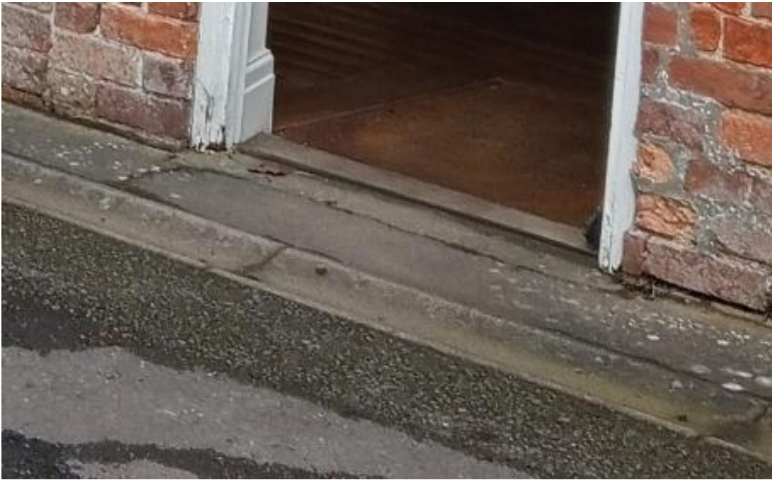
Uneven main entrance
