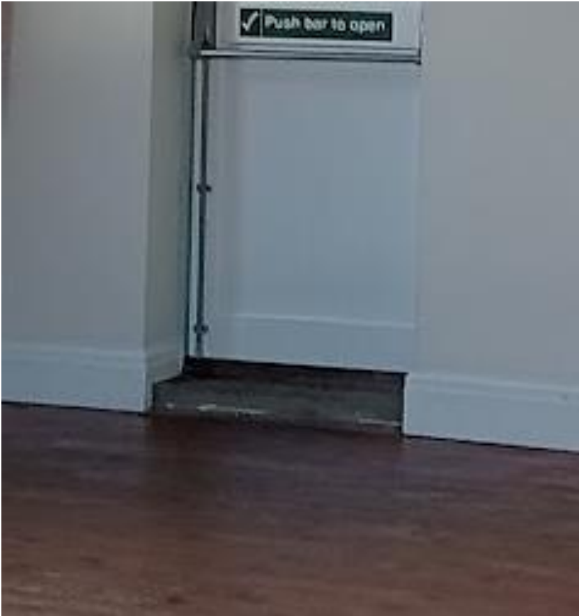
Inaccessible fire exit
